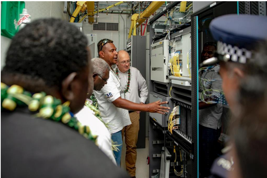
Inside of the cable landing station
